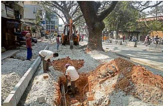
POOR PLAN This picture, taken during 'white-topping' in Basavanagudi, shows how roads and footpaths are built with concrete choking trees.
